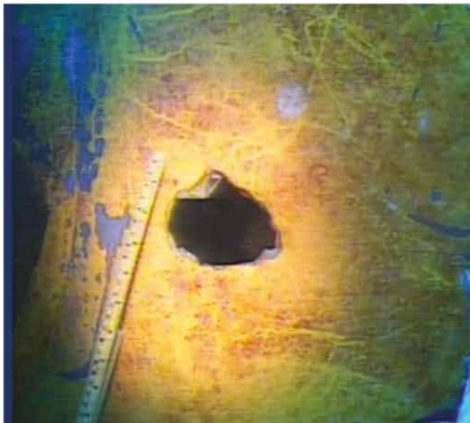
Figure 2. Measurement of the defects.
