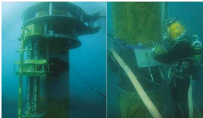
Figure 3. Tape wrapping machine monitored by diver.
