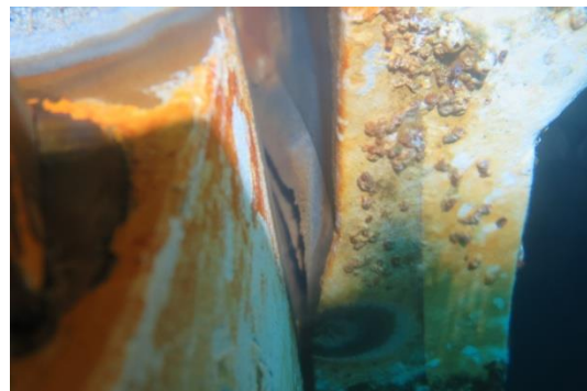
Fig. 6. Damage to the flexible joint receptacle
