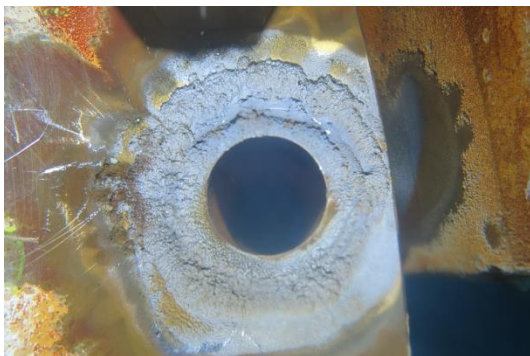
Fig. 5. Damage under leaking nuts (max depth = 1cm)
