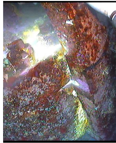
Fig. 2. Leak observed at flange interface
