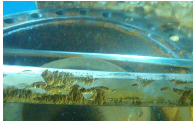
Fig. 23. As-found condition of the BX steel gasket
