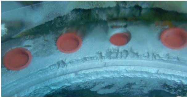
Fig. 24. Example of the groove severe damages on the flexible joint body and receptacle
