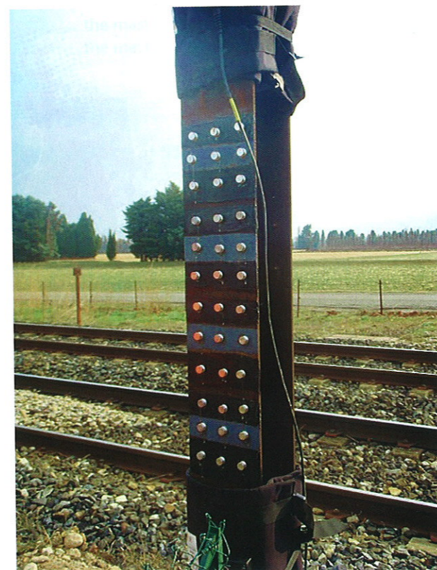
Figure 9: Preliminary study on restoration of a corroded mast made of CORTEN steel to select the most appropriated resin.
