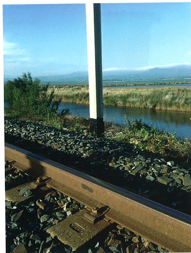
Figure 8: Restored mast on the Narbonne to Port Leucate railway line in the Aude.
