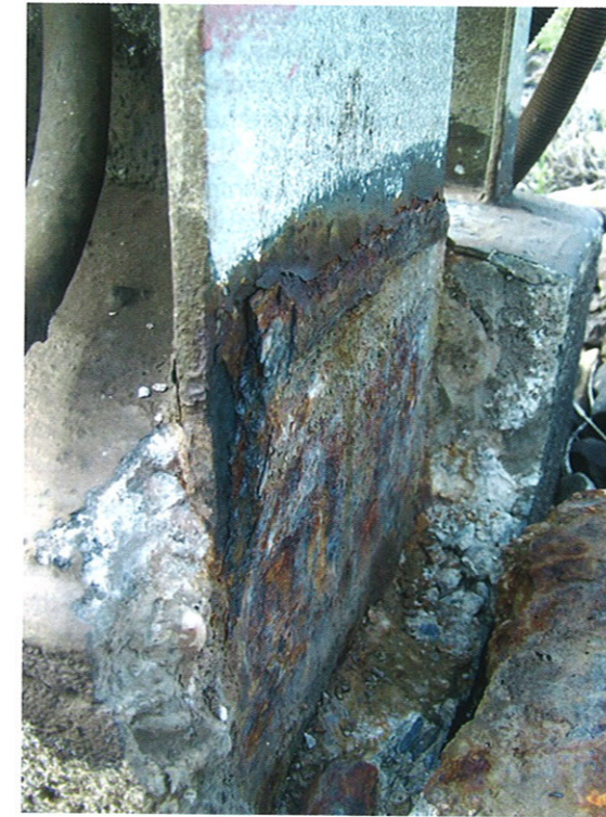
Figure 1: Typical example of corroded mast in French network (photos 1, 2, 3, 5 and Figure 6: SNCF).
