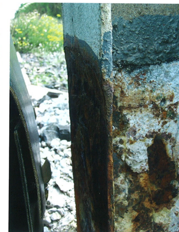
Figure 2: Typical example of corroded mast in French network.
